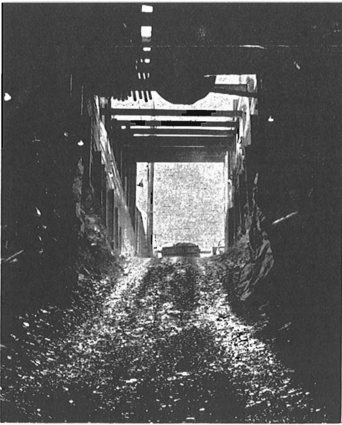
MONTREAL SUBWAY UNDER CONSTRUCTION — Contract No. 1 on line No. 2 (North-South), Berri Street, between Jean-Talon and Jarry Streets. Entrance of the tunnel near Jarry Street.
