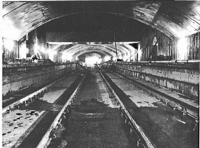
A typical section of a station partly built in rock. This is Crémazie Station on line no. 2. Laying of track was under way when this photograph was taken.
