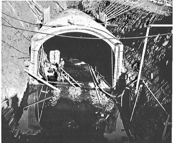
From St. Helen's Island to Notre-Dame Island, on line no. 4, the subway tunnel was built in open cut between two provisional dams closing the south arm of St. Lawrence river.
