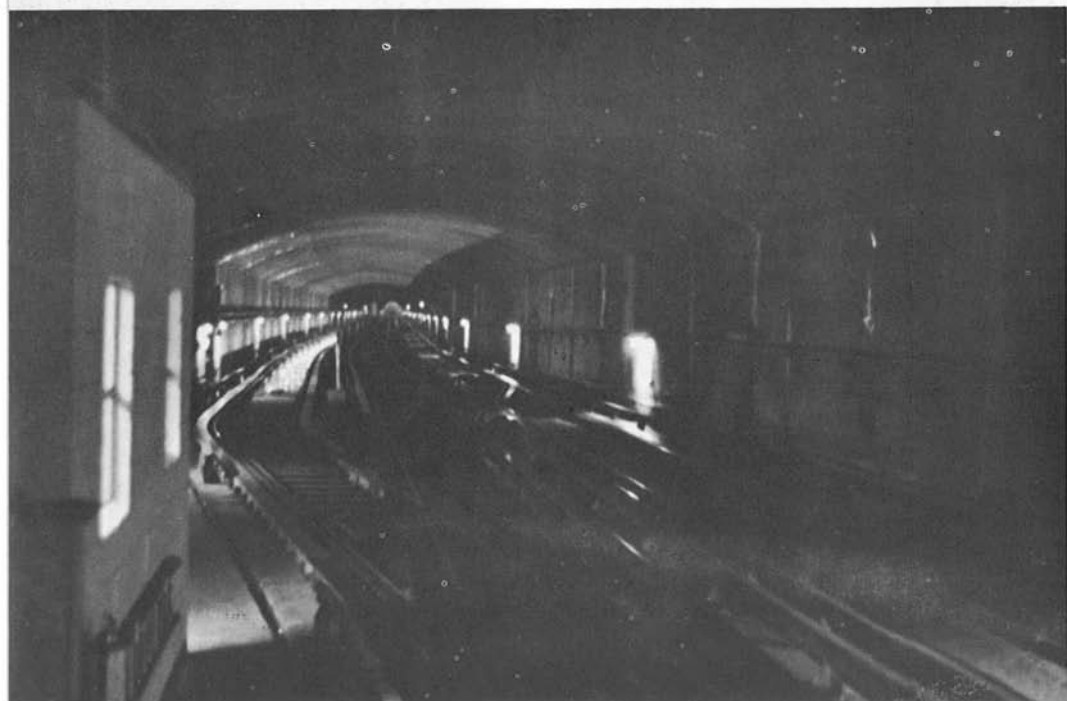
BELOW: Looking north into the tunnels from Cremazie station, a stretch of three-track tunnel can be seen. Two lines on right are the running lines; track on left is the lead to Youville Shops and is fitted with an inspection pit for emergencies. (OSAL)
