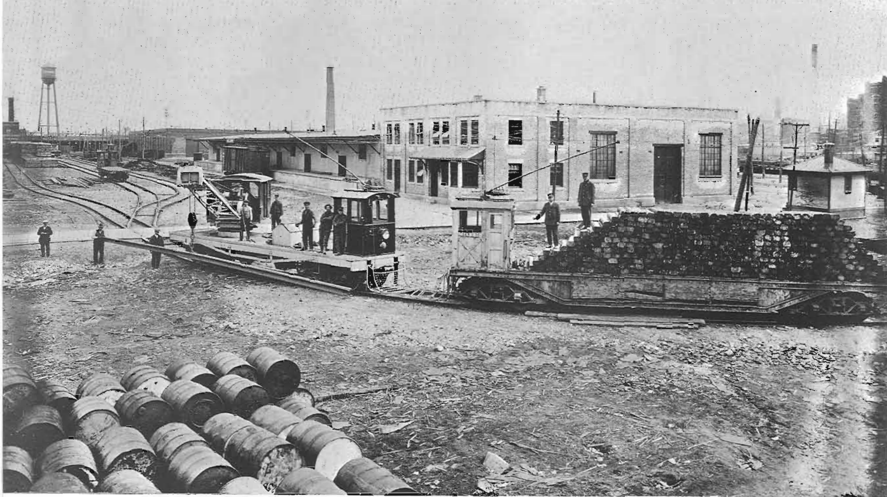
Flat Car 3018 was originally Ballast Car "S". It is shown here delivering a load of ties to Crane W-1 during reconstruction of trackage near St. Denis Carhouse.
