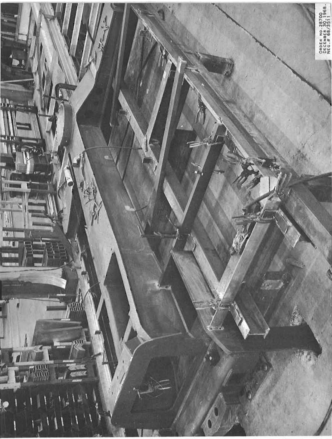
↑ AT CANADIAN VICKERS LIMITED, THE UNDERFRAMES FOR THE NEW CP RAIL GALLERY cars are being assembled in a jig before being welded. Photo by CP RAIL. → AN INTERIOR VIEW OF THE COMPLETED GALLERY CAR STRUCTURE-STAGE 8 IN the construction process, followed by a picture of the first car structure in the "squeeze" frame. The white areas are "Stress-coated" to show the areas affected during the test. Photos CP RAIL.
