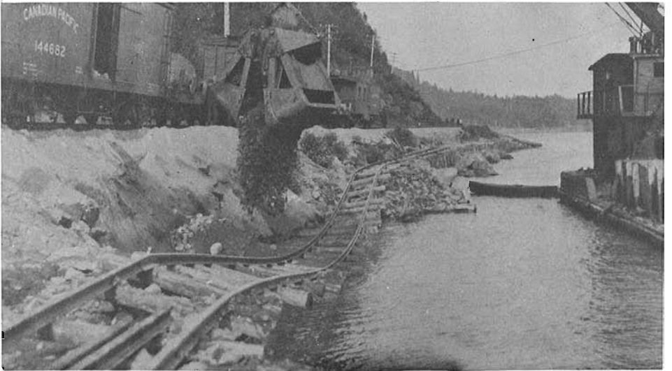
Even after completion of the grade workmen had to often return to repair flood damage to newly placed fill. Firstly a slide at Red Rock being repaired by a clam shovel aboard a barge, then two photos of serious washouts along the line. All photos in this series courtesy of the author's collection.
