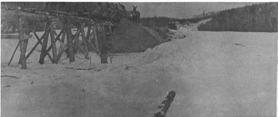
Animal power pulling narrow gauge lorries was the order of the day as workmen dug through this clay cut at mile 86, the lorries were transferred to locations requiring fill as noted in the second photo. View of yet another extensive cut under construction near the town of Nipigon.
