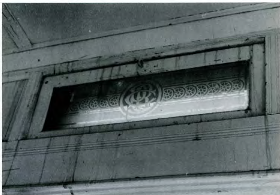
An example of the decorative clerestory windows, some of which are hidden by wood sheathing. The pattern apparently depicts a stylized locomotive wheel and CPR script.
