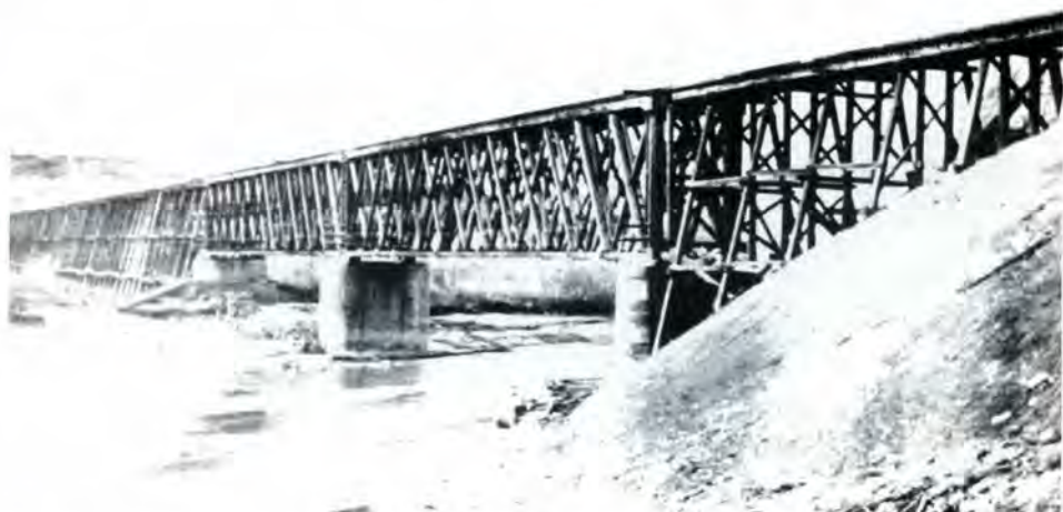
St. Mary River double truss. The far pier is the only one standing today, the other two having fallen over.
