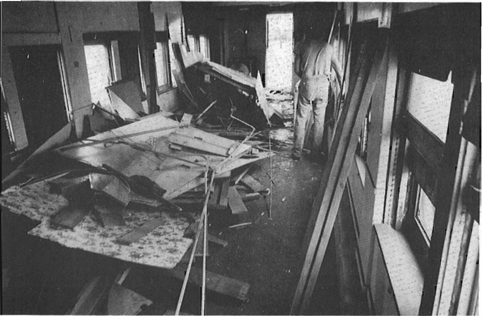
If you think the exterior of the car requires work, this was the scene inside. The refuse on the floor is what was left after the removal of the lateral partitions that were required for service as a boarding car.
