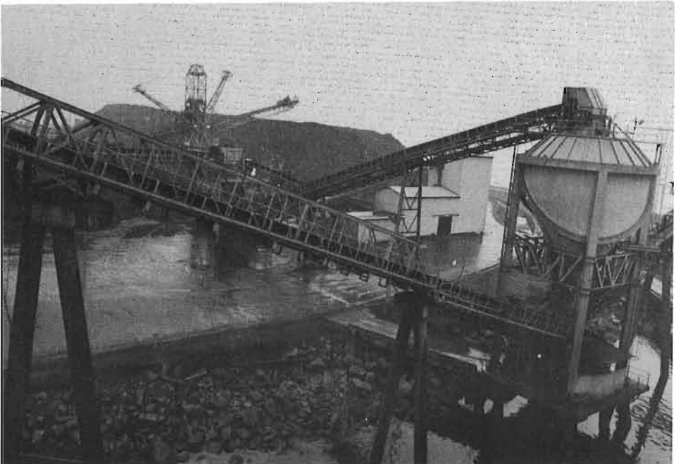
Assortment of conveyor systems within the stockpiling area. Coal arriving from a unit train can be distributed to any one of four stockpiling areas, or directly to the shiploading system. Hopper and delivery systems are flexible and allow changes in stockpiling requirements.
