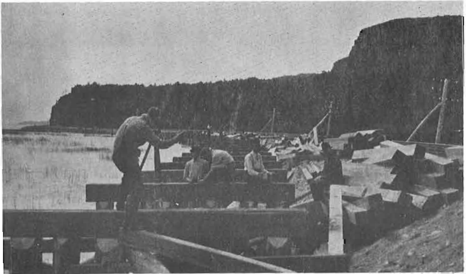
Photos showing the construction of trestle cribwork at Red Rock and the digging of a cut near Nipigon, Ontario for the Canadian Northern Ontario Railway. Both photos courtesy Mr. A.J. Isbester.
