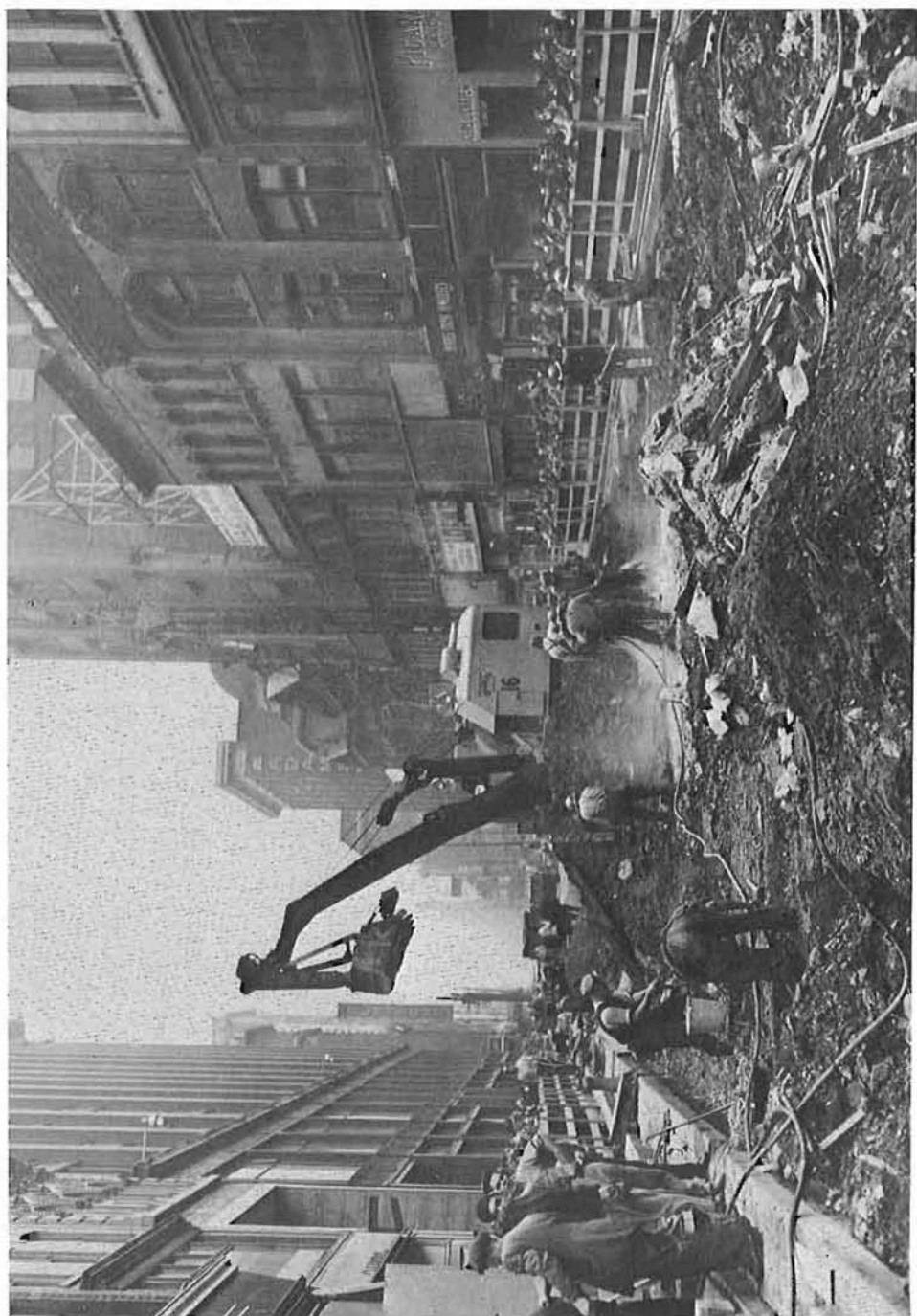
The start of excavation work for the Yonge Street Subway, circa 1950. Lots of hand work was involved because the exact location of services was unknown. Photo courtesy TTC.
