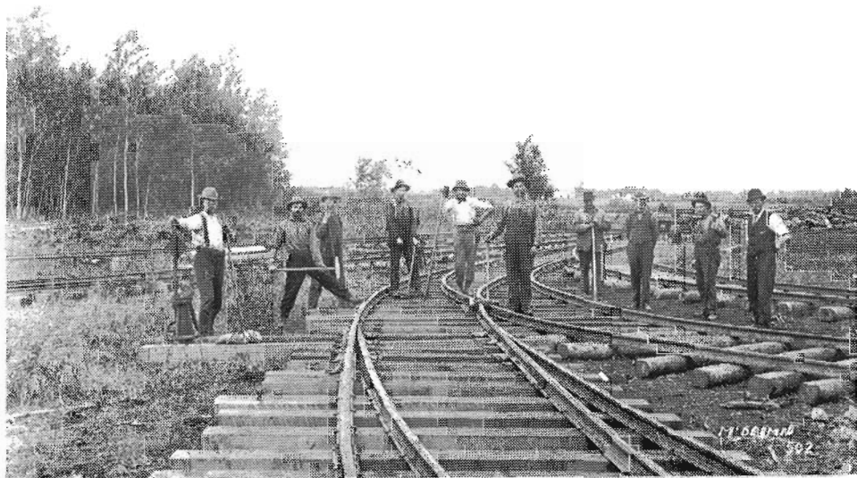
VIEW OF THE TRACKS GOING INTO THE CAR HOUSE. Photo taken from the car house. October, 1913.
