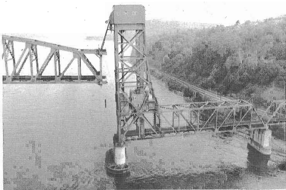
LIFT SPAN STRETCHED out of alignment with South tower
