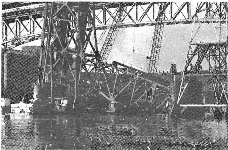
THE CRANE BARGES ARE NOW IN POSITION ready to begin lifting the damaged span
