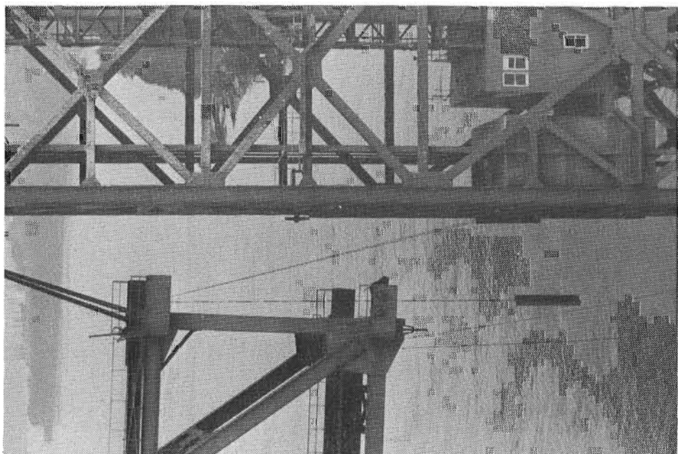
A CLOSE-UP VIEW SHOWING HOW THE LIFT SPAN was stretched out of alignment with the South tower
