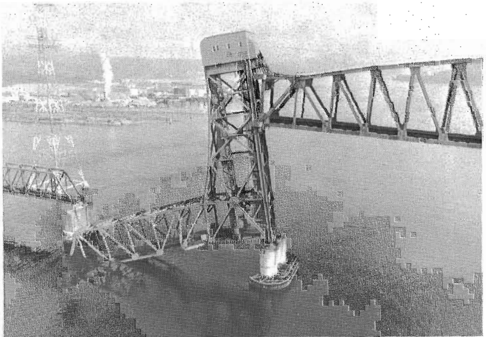
A VIEW OF THE DAMAGED TOWER soon after the collision. This view will give some idea of the problems faced in repairing the bridge
