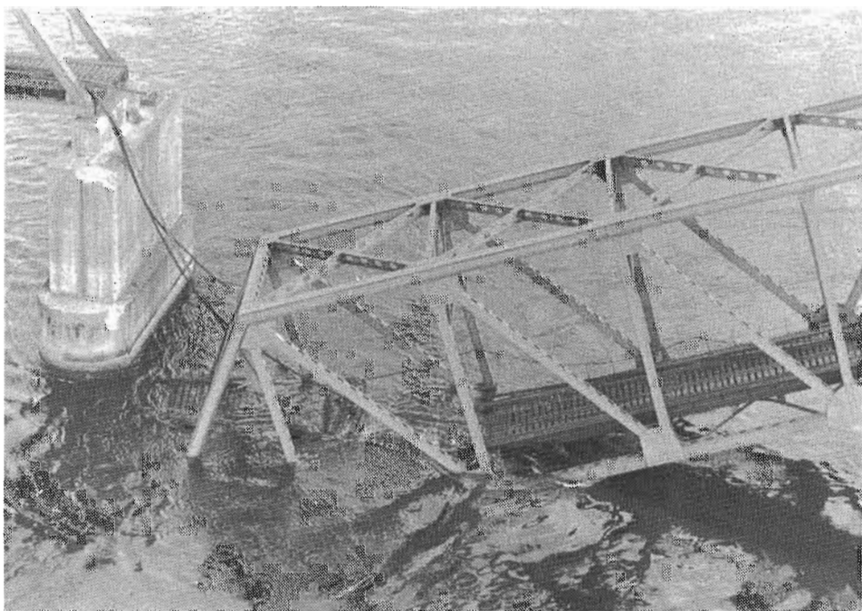
NORTH END OF STATIONARY SPAN after being knocked from its anchor pins
