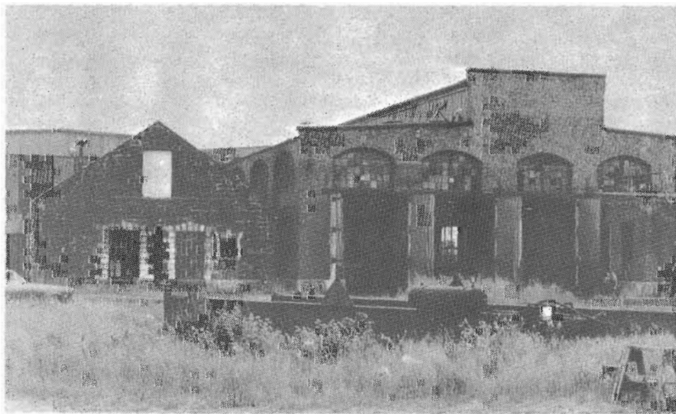
RAILWAY SHOPS IN CHARLOTTETOWN. The three stalls in the main building are the areas where repairs are done.
