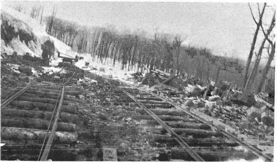
THE PARTLY-COMPLETED RIGHT OF WAY as seen on March 1 1928 looking Westward from just below the summit, near where the previous photo was taken. The temporary light tracks are for carrying debris from the excavation site.
