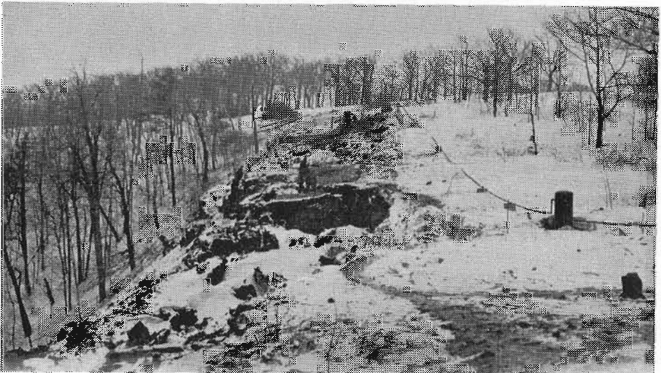
THE EASTERN APPROACH TO THE TUNNEL as seen on March 10 1928, looking Westward before the excavation began. A comparison of this view with one taken of the completed line shows the tremendous amount of rock which had to be removed. At this point a deep cutting was made into the mountainside leading up to the tunnel. The pipe line running to the right of the future cut is to carry compressed air for the drills
