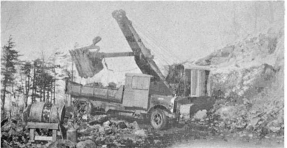
TWO MONTHS AFTER WORK BEGAN the excavation had reached the summit, about half way between the loop and the tunnel. This view was taken on February 28 1928 looking Eastward, and shows Cooke Construction Company's power shovel loading a truck with blasted rock.
