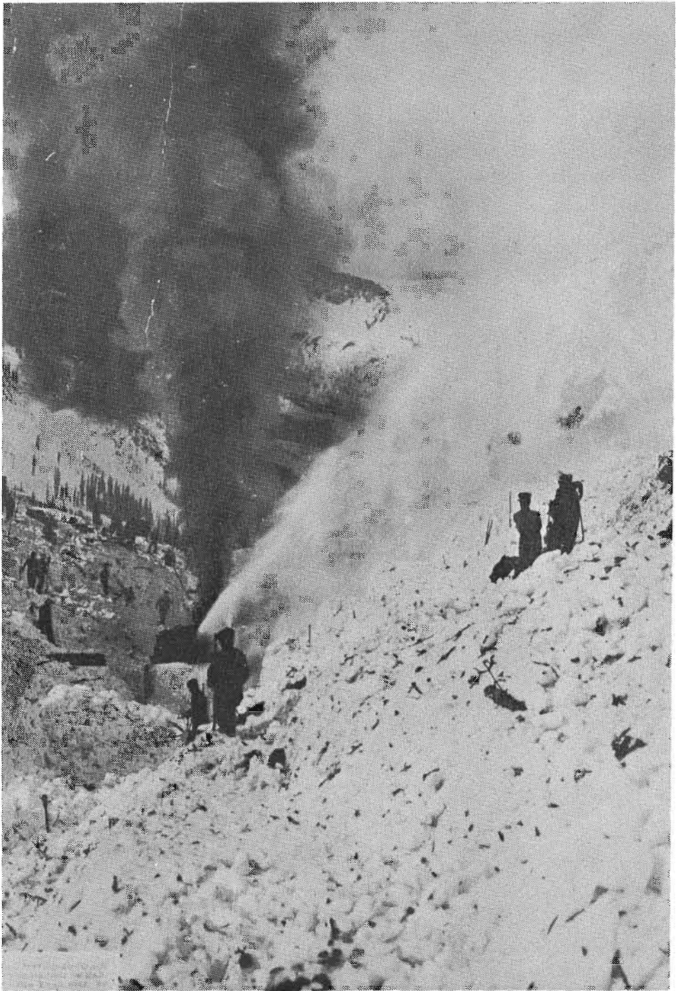
THE ROTARY IN ACTION WAS A SPECTACULAR SIGHT as can be seen from this photo taken in 1910. The scene is probably Rogers Pass after a disastrous snow slide. Pieces of broken trees mixed with the snow were always a hazard to operation of rotary plows.
