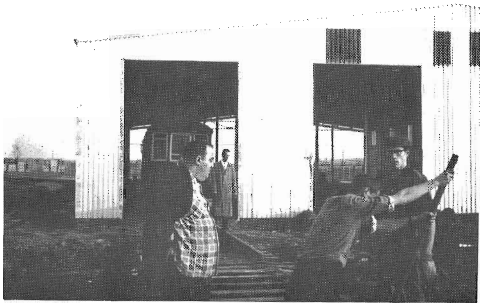
AS WINTER CLOSED IN there was a race to get as much equipment as possible under cover. There was no time to build switches, so as a track was filled the outside track was moved bodily over to allow construction into the adjacent bay. These two views show the track being jacked over on a Sunday afternoon, December 2 1962.
