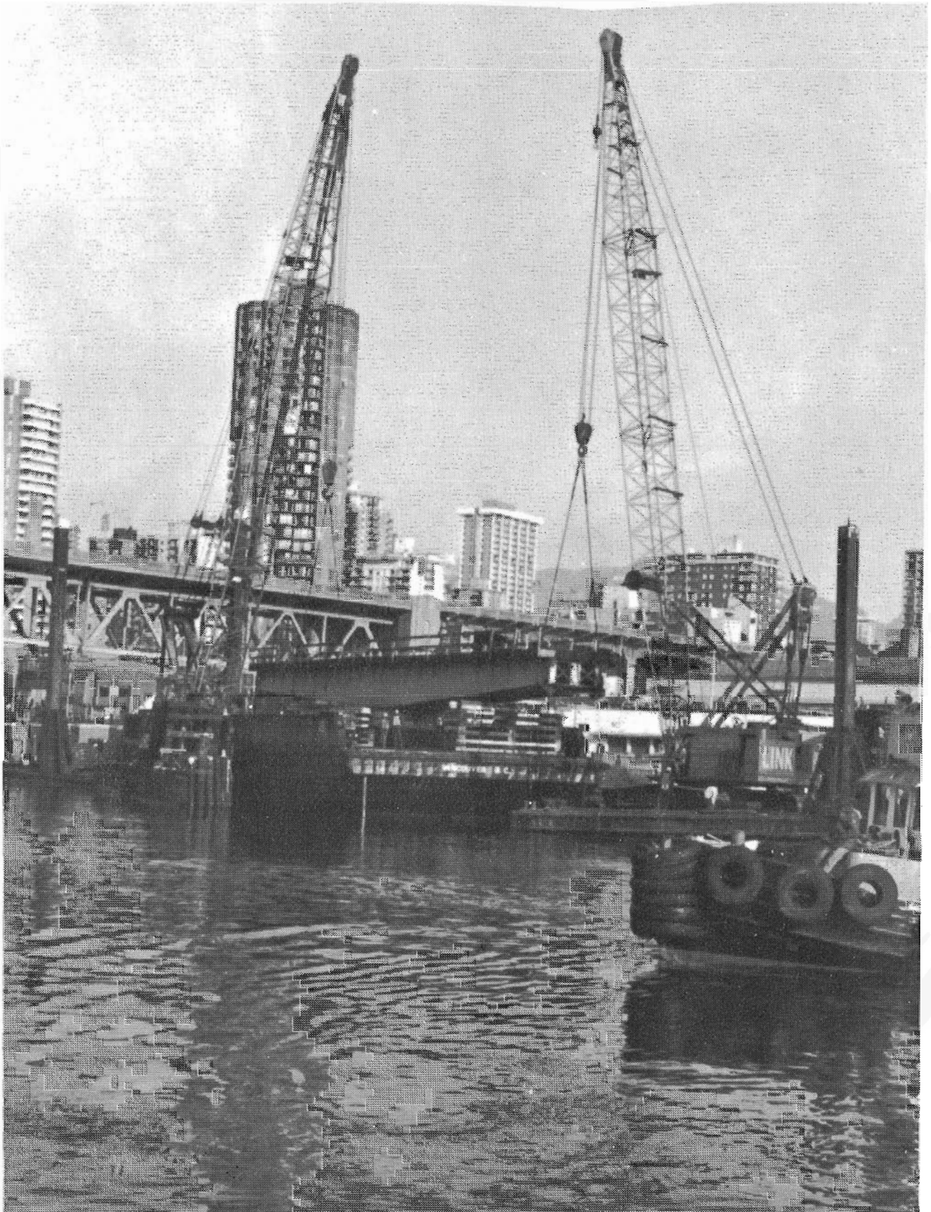
Two barge-based high cranes lift the moveable span from its pedestal. Photo courtesy of Norris Adams, Vancouver
