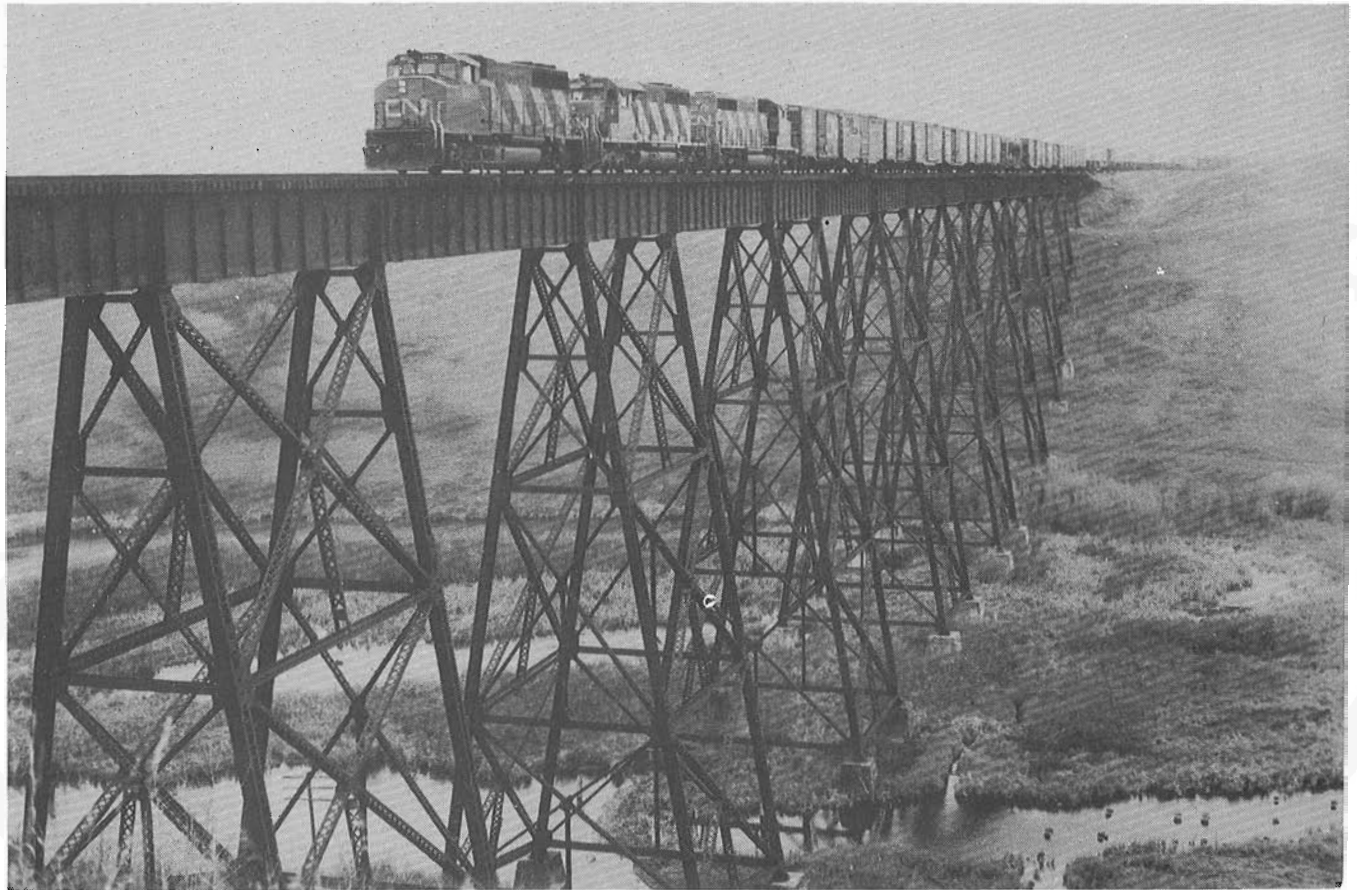
The highest, though not longest, bridge on the Rivers sub. is over Cutarm Creek, near mile 234, just west of Gerald, Sask.. Opened to traffic by CNR in 1925 it is 1,152 ft. long with maximum height of 135 ft.. Under a low fog on Oct. 17, 1982 a GP-40 and two SD-40's 9625-5102-5279 are making fast time with symbol freight No. 301. A large colony of beavers, shunning a man-made dam a little upstream, have built one of their own a little downstream. Apparently the rumble of the trains doesn't bother them as one of their lodges can be seen between the bridge footings at bottom center of the picture. I regret I have never been able to find a picture of the earlier bridge at this location. L.A. Stuckey photo
