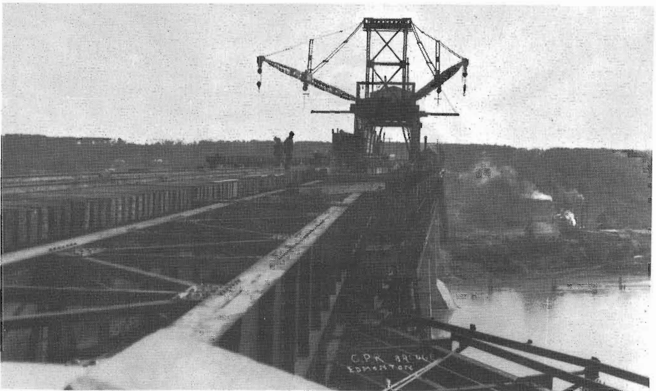
This is a good view showing the traveller used in the construction. It was arranged to erect not only the main spans but also the other spans without falsework. The rigid arms are extended to counterbalance the high winds in the valley. The sidewalk and roadway are below.
