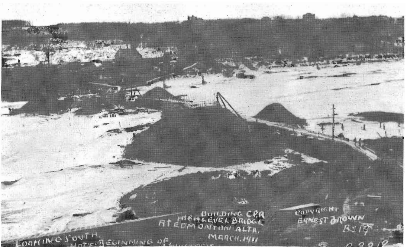
The pier excavations are well under way in this view looking south in March 1911. Almost ready for the frameworks for the concrete pouring.
