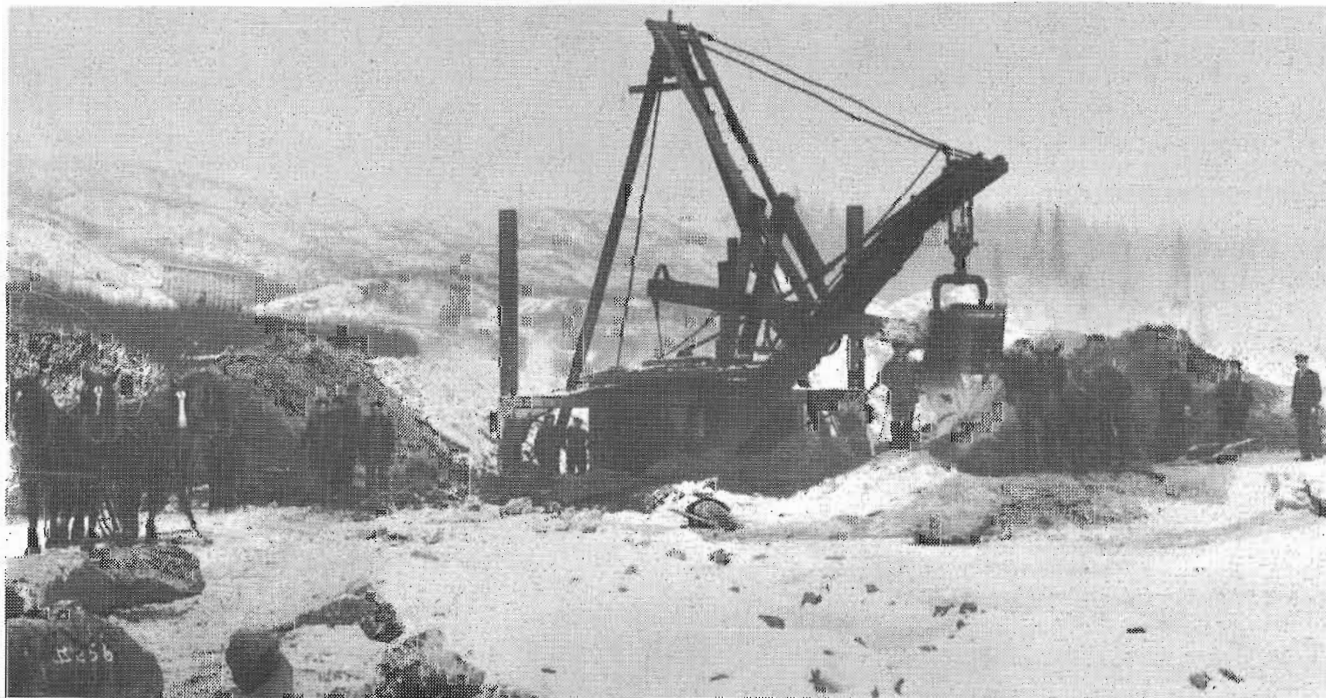
The excavation for the first pier of the high level bridge taking place during the winter of 1910 - 11. Provincial Archives of Alberta B3337.
