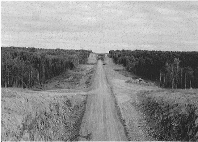
On concession road 5 viaduct, looking east, in the distance, concession road 6's viaduct.
