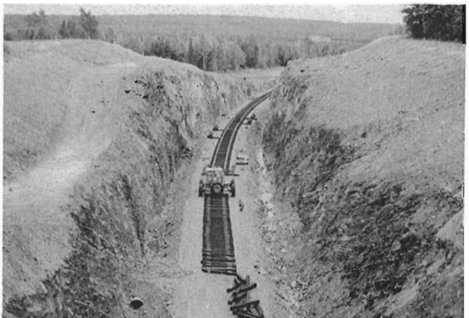
On concession road 6 viaduct looking eastward, the clearing in the distance is the right of way after a big curve, it is the week-end rest.
