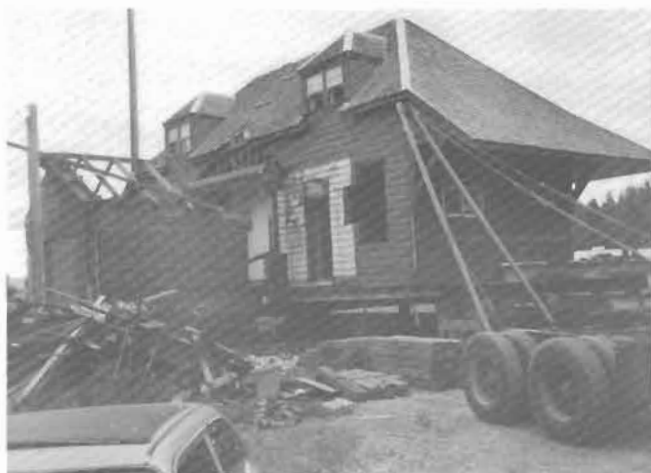
The Elko station in July 1987. It has been separated from the back addition, has been lifted and is being moved off its old foundation.
