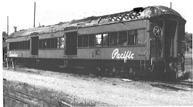
Former CP 80-foot baggage car, now the property of Salem and Hillsborough R-R. in the process of being repaired (new roof) and converted to an open tourist car.
