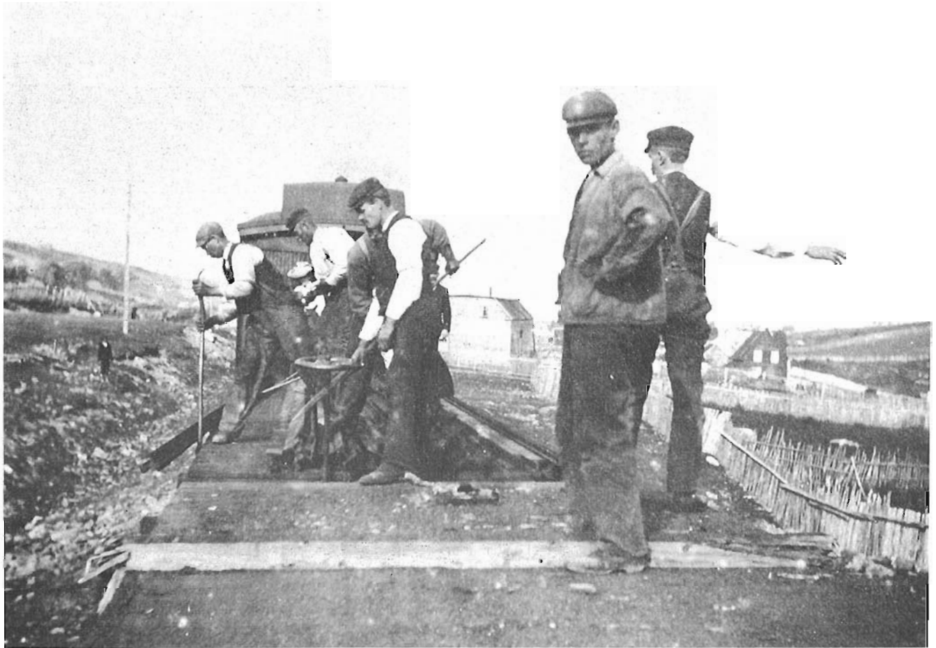
A work crew unloading rails from a flat car on the Newfoundland Railway around the turn of the century. Provincial Archives of Newfoundland and Labrador.
