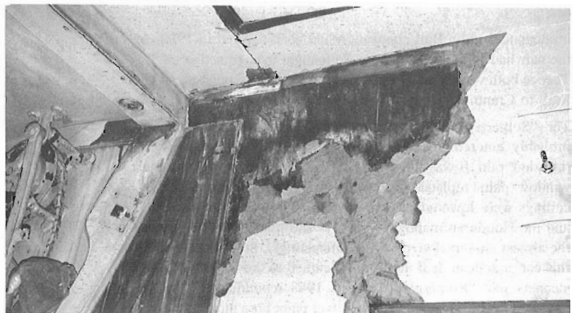
As this view, taken on December 13, 1991, of "Somerset" / "Travers" shows, the starting point can often be close to heartbreak!
