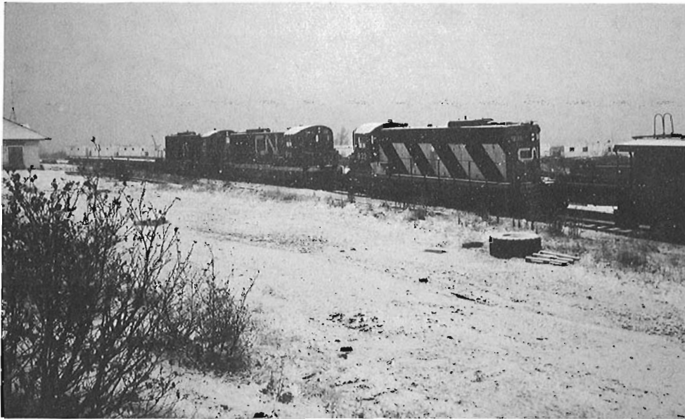
The last days of the Clarenville rail yard as seen on November 12, 1990. Shown here are locomotives 937, 932, 914, following the end of dismantling operations. All main line track has been removed in both directions.
