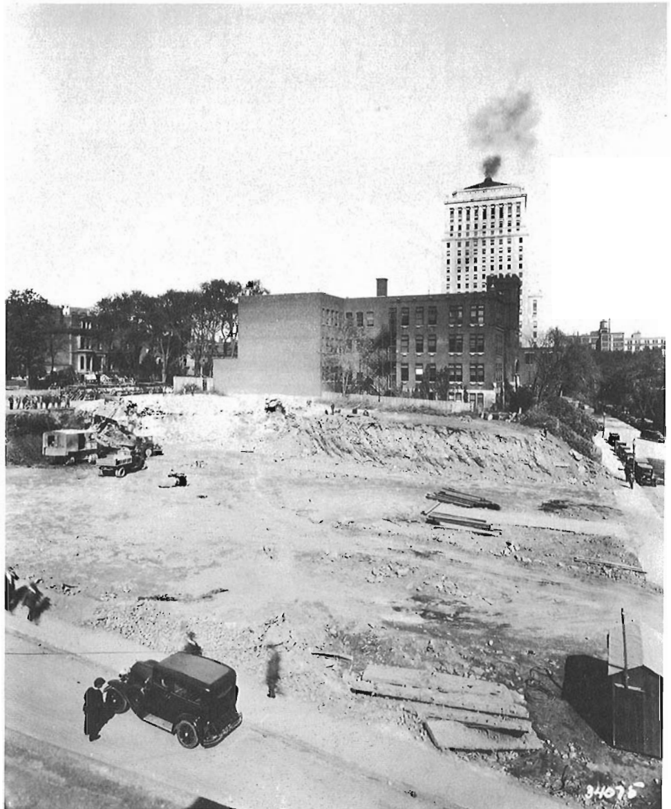
The start of the excavation for Central Station as photographed in 1929. The view is taken looking east, with Lagauchetiere Street on the right. Notice that some of the old houses on Belmont Street (extreme left) were still standing.
