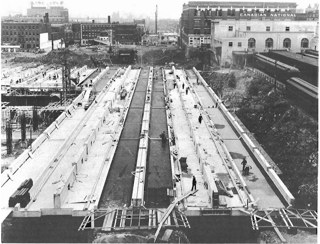
Constructing the platforms. August 4, 1939. View looking south. Note the old Canadian Northern tunnel terminal on the right. Canadian National photo No. 42726-2.
