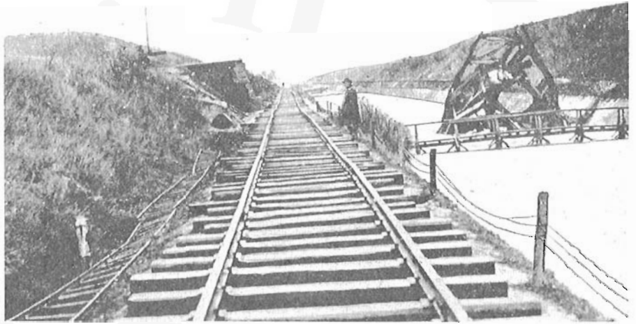
A section of newly laid track along the path of the Canal du Nord in France on November 27, 1917. CRMW, September, 1919.
