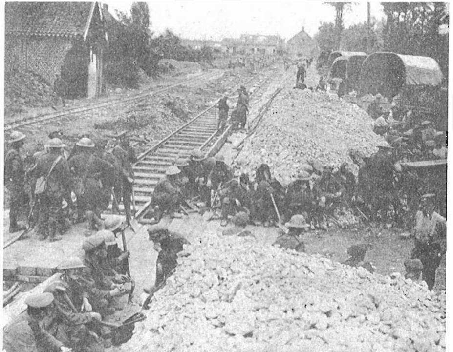
Canadian Railway Troops working on a standard-gauge line running alongside a narrow-gauge light railway. CRMW, December, 1919.
