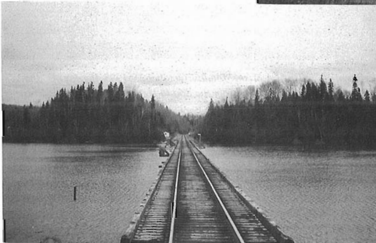
LEFT: Nearing the end of the longest stretch of track covered in one day, the Sperry crew crossed a branch of Oba Lake, at Woods Camp, on October 25, 1993. Near this spot, at Oba, the main line of Canadian National crosses the ACR. The work for the day ended at Oba.
