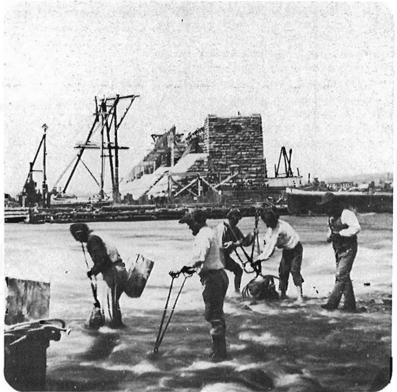
Breaking up the old coffer dams during the summer of 1859; a difficult job in its own right. NPA photo No. 7023.
