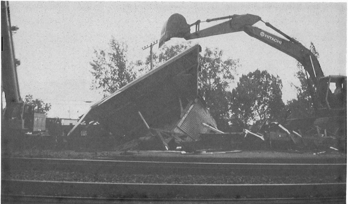
A sad end! The demolition of Val Royal station on June 5, 1995, less than three days after the end of service of the old CN electrics. Such was the end of a site beloved by railfans for many years.
