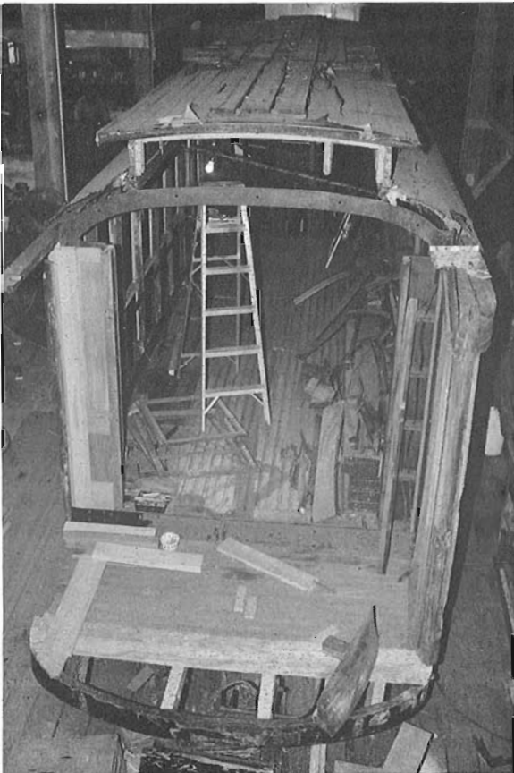
Dismantling of the rear vestibule was complete by December 10, 1988, when this photo was taken, and a new subfloor was under construction. High Iron photos 356-95-5e.
