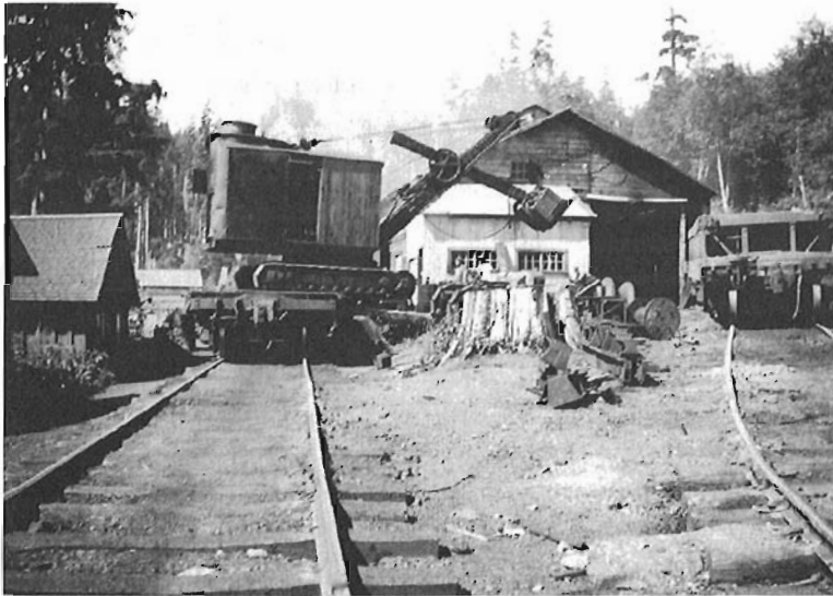
Allison found a power shovel very useful in building the railway in swampy areas. This photo is behind the shop building at camp and shows the Marion shovel being loaded onto a heavy flatcar. The wooden ballast car at right was one of three used on the operation. -Stan Unsworth photo, Author's Collection
