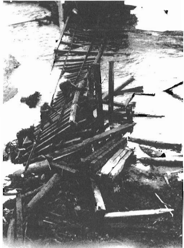
No. 72787 - CNER, the old sections of the original bridge over the Bear River were sawn up & pulled down to allow reconstruction of a new bridge to replace it. Note the men climbing on the twisted rails over the rushing river
