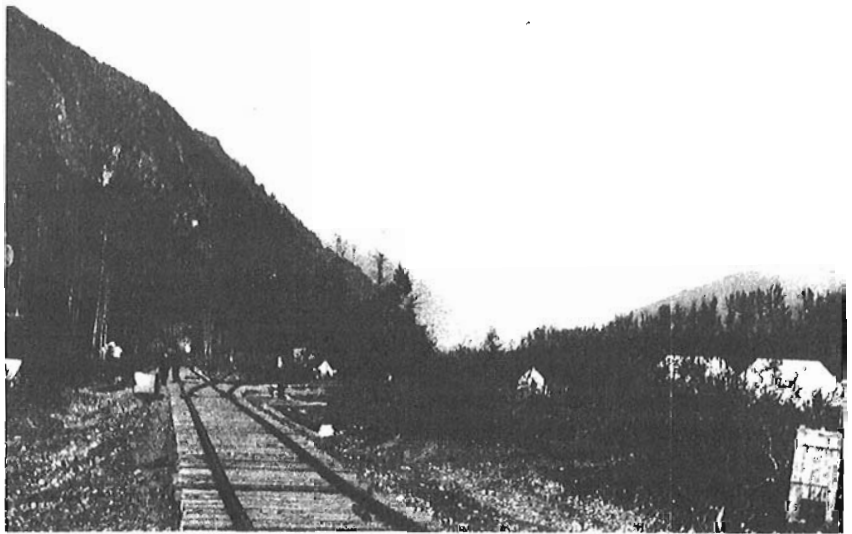
No. 7483 - PCSL First Rails Laid (1911). Note: All photos are from the Public Archives of British Columbia. The number at the beginning of the caption is the P.A.B.C. number.
