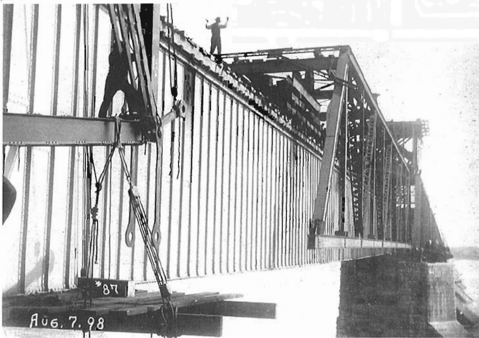
This spectacular view was taken near the centre of the bridge on August 7 1898, as the construction of the steelwork neared its completion. A temporary movable structure has been built inside the main spans until the much larger centre span is finally in place. National Archives of Canada, photo PA-202510.
