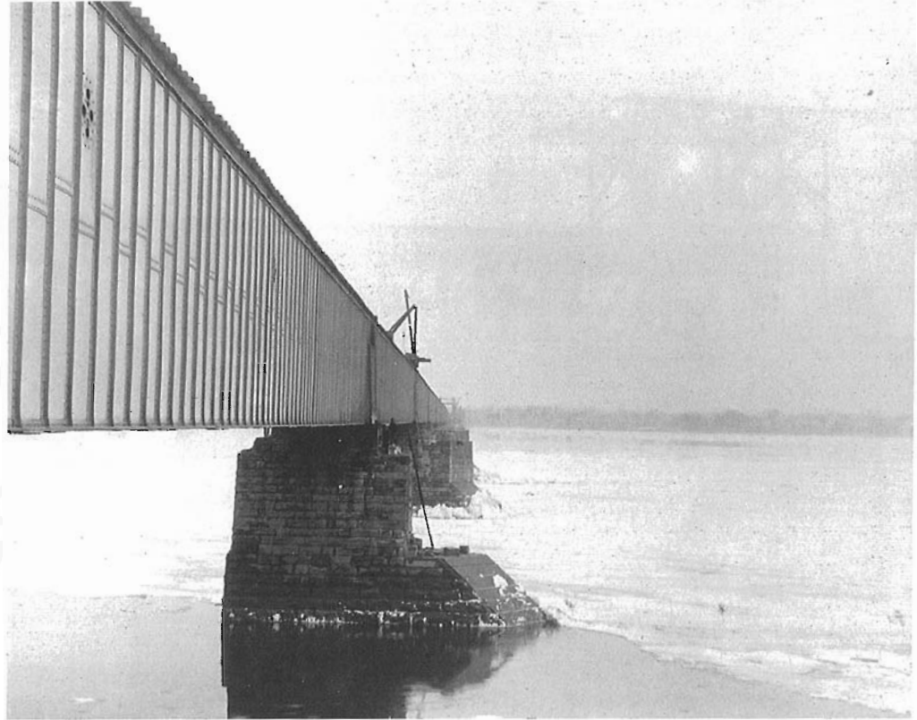
ABOVE: In March 1898, one of the piers is being prepared for widening by building up the upper portion of the pier to floor level. Note that the lower portion of the pier did not have to be widened. The pier in the background has already been partially built up. National Archives of Canada, photo No. PA-202500.
