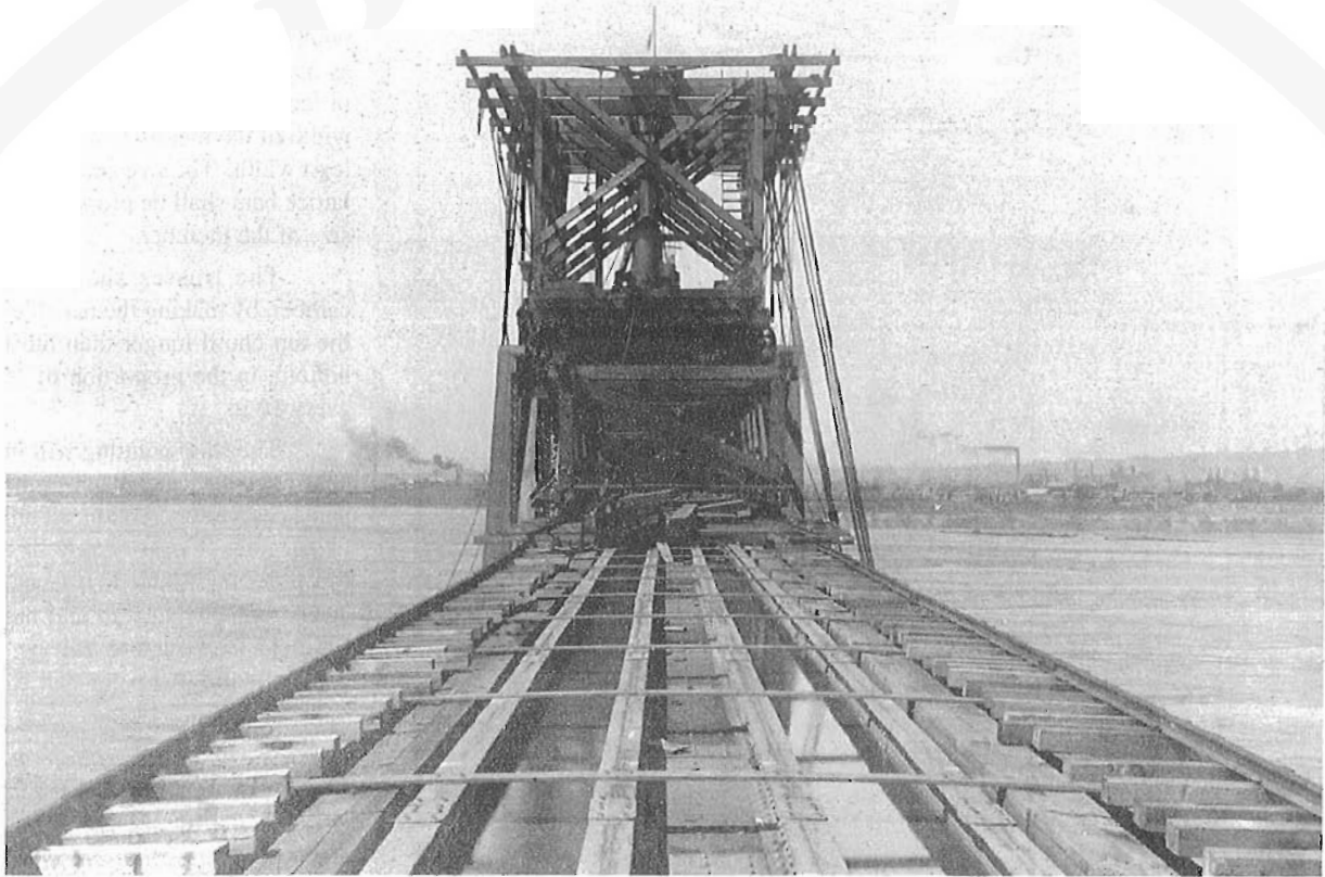
The heavy equipment used to hoist the parts of the new spans. The span behind has been completed. Judging by the position, this appears to have been in May, 1898. Note the skyline of Point St Charles in the background.
