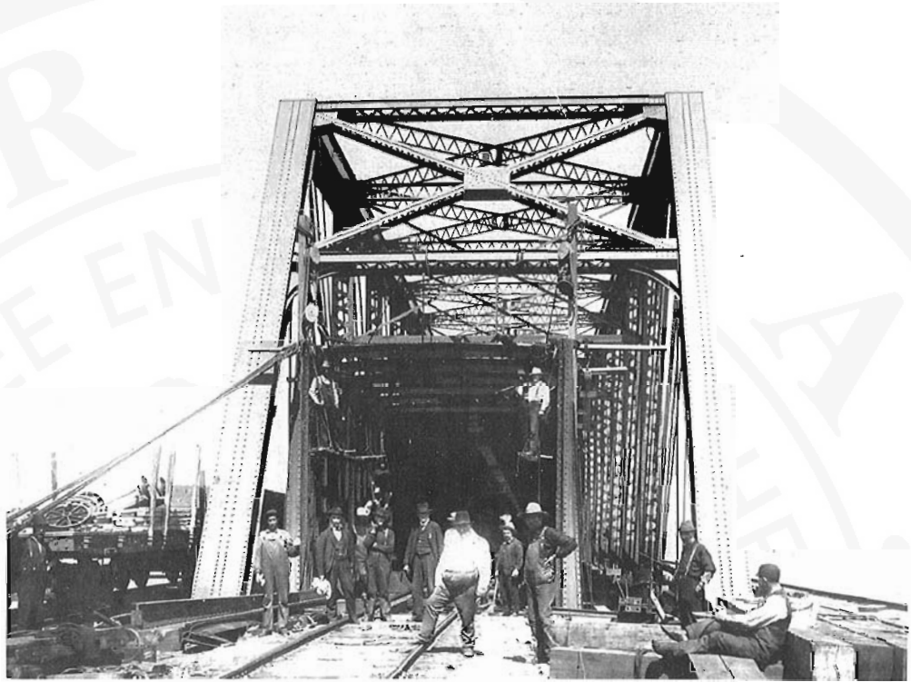
It's now July 5 1898, and a group of workers take a brief break to pose for the photographer. There is still much work to be done, however. Three spans remain to be built, including the all-important centre one. The old tube is still in use, but some of its roof has been removed and in a few months it will be dismantled. Note the temporary tracks on the side roadways; used to carry supplies without tying up the main line.
