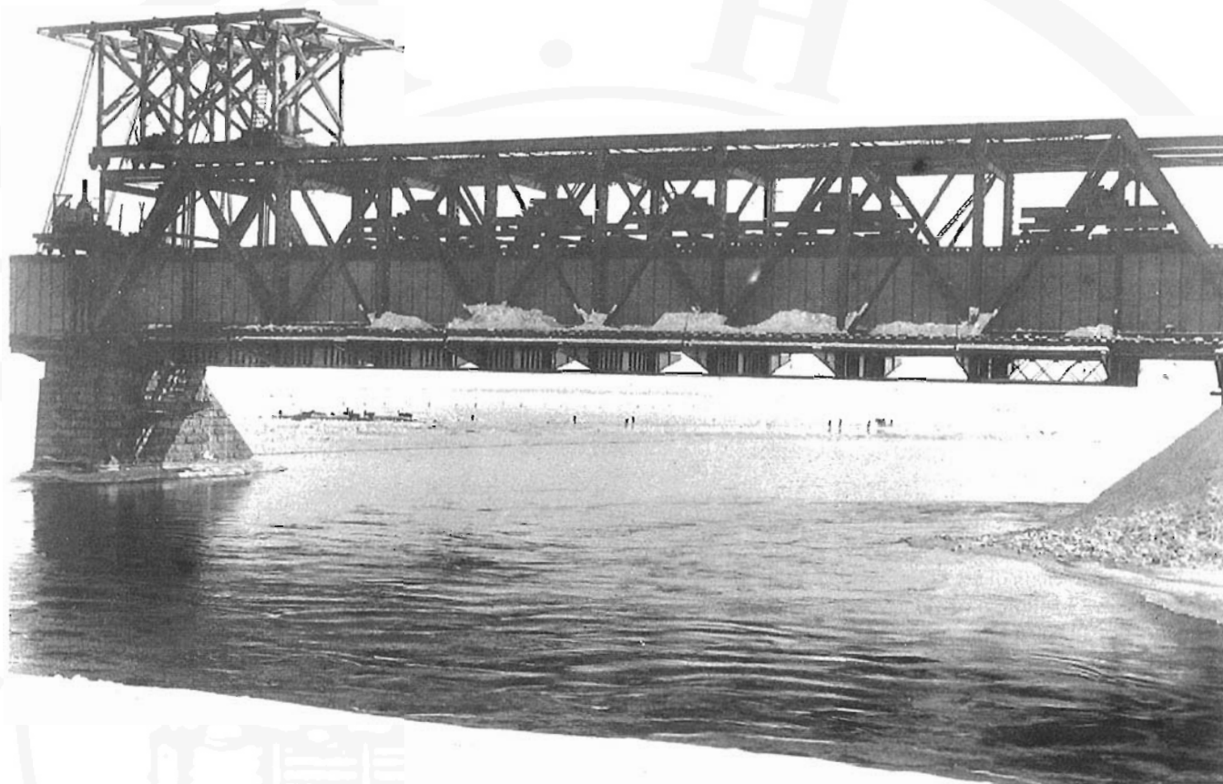
The completion of the first new span; March, 1898. Note the vertical steam boiler on the left. This supplied steam to the hoisting machinery, and powered the traveller. National Archives of Canada, Photo PA-202504.
