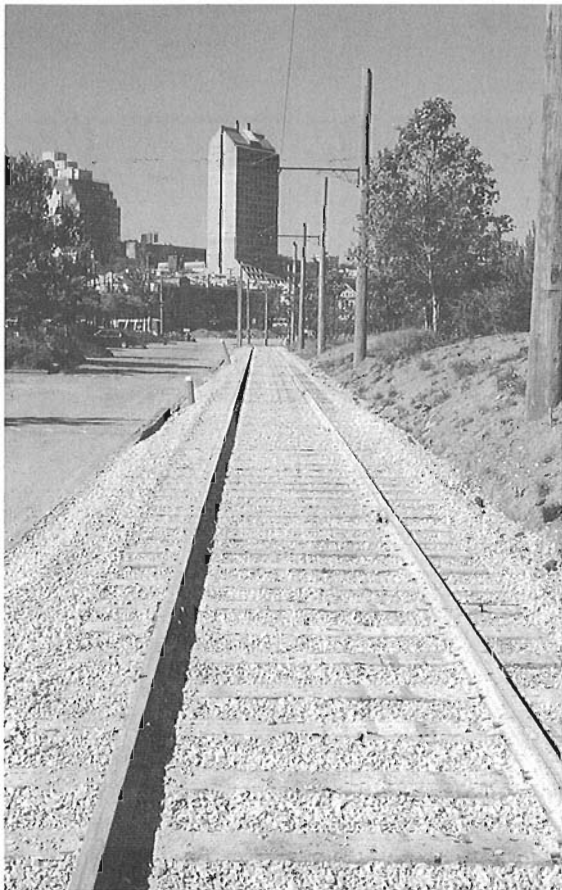
Line shot showing the quality of rail and overhead construction. Photo by Peter Murphy
