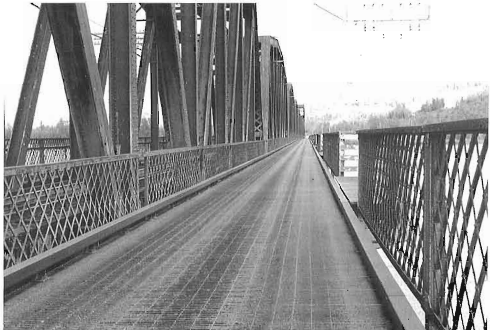
View of eastbound cantilevered roadway in 1996. This roadway has not been used by the public since 1987. Photo by the author
