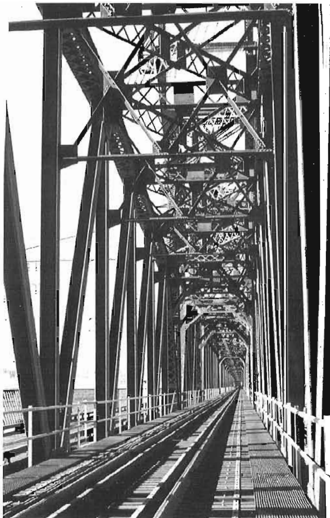
Interior view of the spans, looking west, October 1999. Photo by the author.
