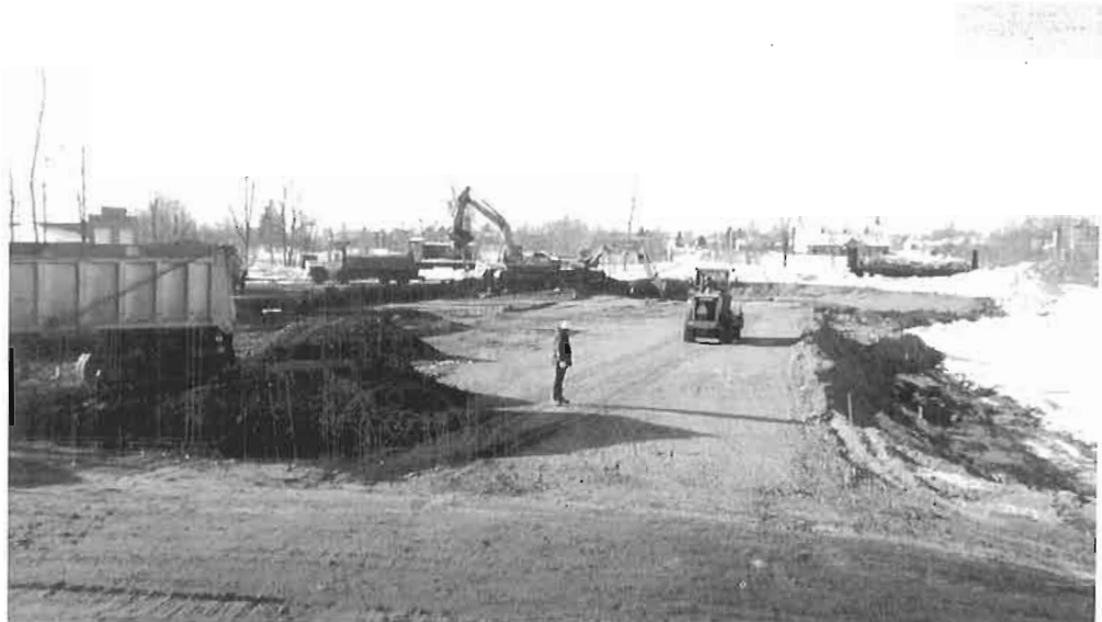
Levelling ground for the new display building. View is from the back to the front of the future building.
