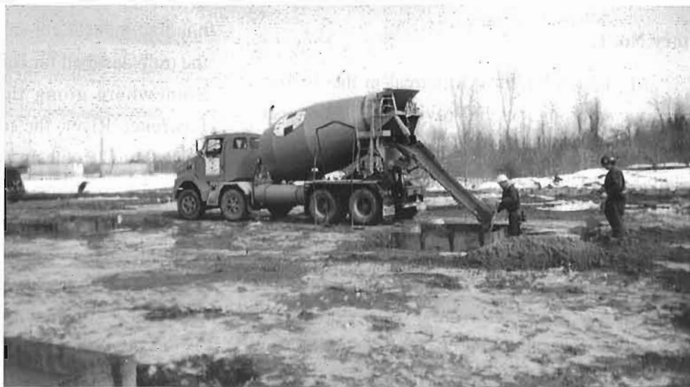
Pouring one of the foundation footings for the new ExpoRail exhibition hall.
