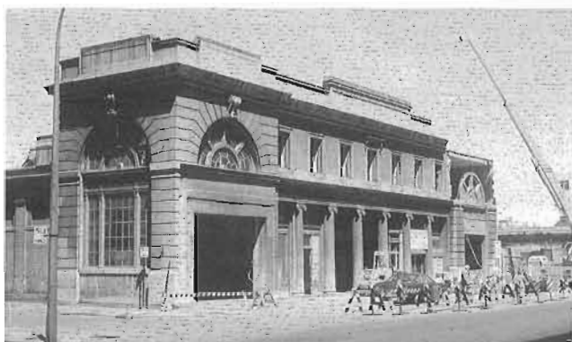
Craig Terminus being demolished on May 17, 1980. The architectural items, carefully removed, still exist, but have never been used.
