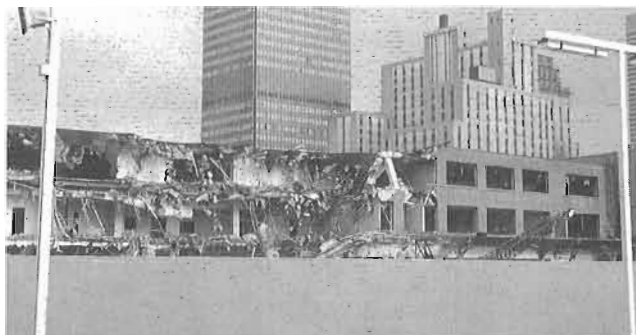
The demolition of the 1953 express wing of Windsor station (seen here on July 25, 1972) led to speculation that the entire station was doomed. However the main portion of the structure was preserved and renovated. The Laurentien hotel in the background was torn down in 1977.
