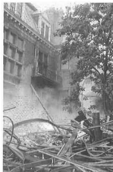
Heritage preservation suffered a heavy blow with the demolition of the Montreal mansion of Sir William Van Horne, the builder of the CPR. Here we see demolition under way on September 8.
