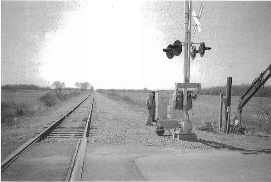
A view west along the CASO line at Wellandport Road (Montague) on April 28 2001. A CPR work crew installs and reactivates level crossing equipment in preparation for the line reopening.
