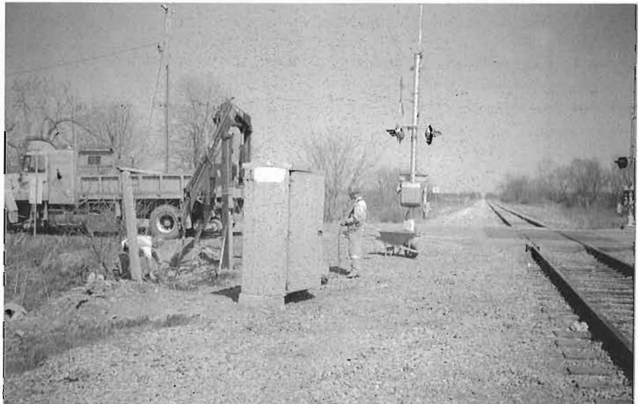
Looking east at the same place on April 28 2001. Another view of the CPR work crew installing and reactivating the level crossing equipment.
