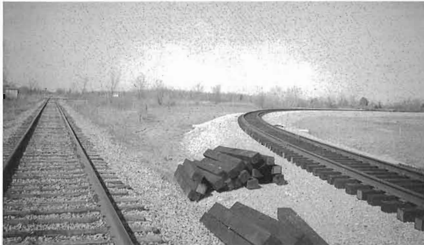
Looking north along the alignment of the ex E&O line on April 28 2001. The CASO line diamond is visible in the distance. Construction work on the new connecting curve at the right remains to be completed.
