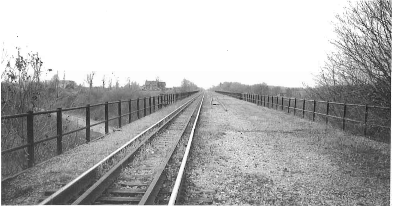
Looking west across the Kettle Creek viaduct west of St. Thomas on November 27, 1999. The sheen on the rails indicates that this stretch of the CASO line hosts a limited local freight service. Note the lengths of 127 lb. continuous welded rail from the lifted westbound main still lying on the trackbed.
