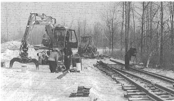
Installation (by Coyle Inc.) of one of three switches on the Candiatic Spur to permit rail access to the Exporail pavilion. Photo by Peter Murphy.
