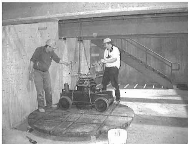
The author and Kevin placing the wheel jack. (GH) L'auteur et Kevin mettant le chariot en place. (GH)
