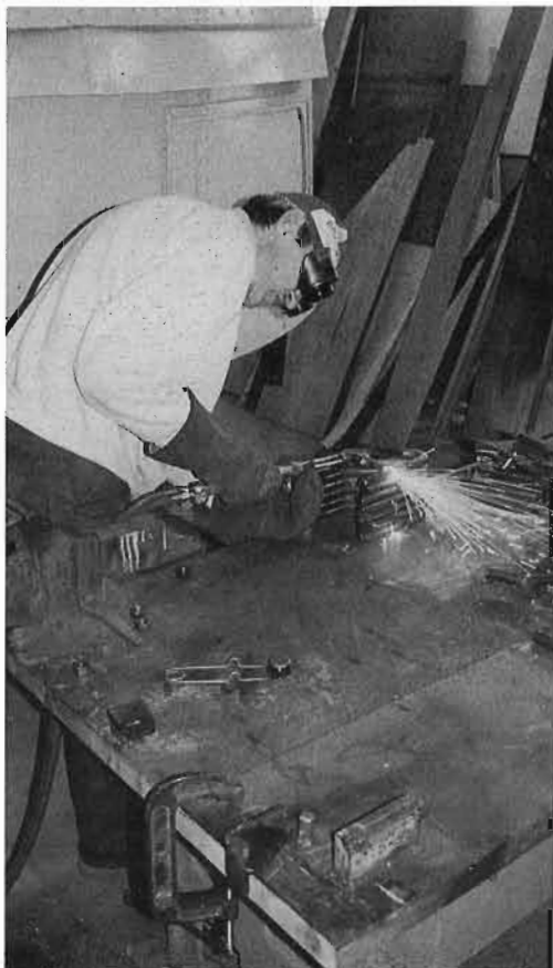
Jean-Claude Hutchison fabricating the brackets to tie the rails to the beams over the pit. (PM)
