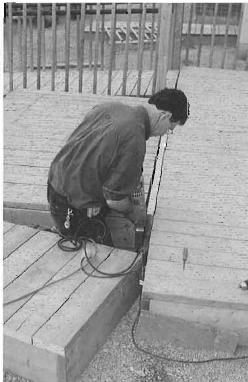
Jacques St. Gelais installing temporary wooden platforms and wheel chair access ramps outside the main doors of the Exporail pavilion. (PM)
