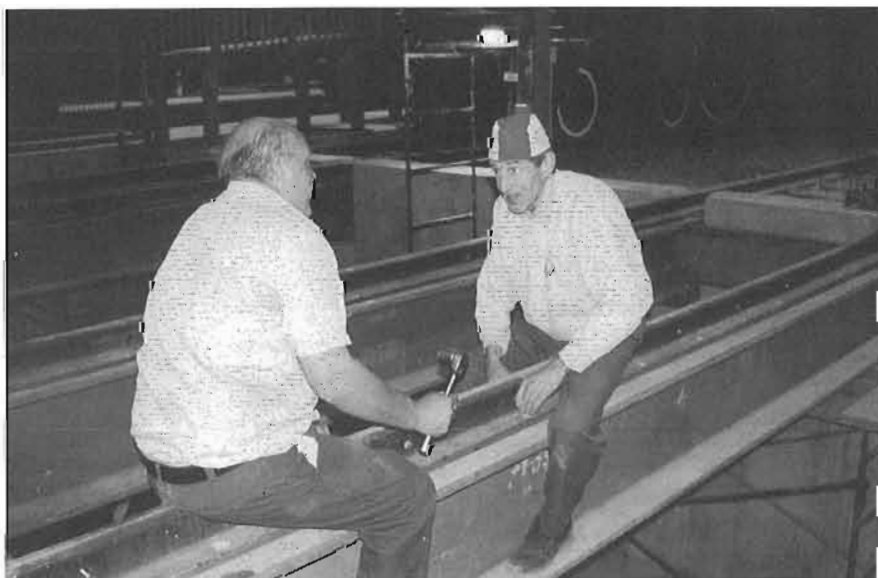
Charles de Jean and Jean Claude Hutchison installing the brackets to tie the rails to the beams. (PM)
