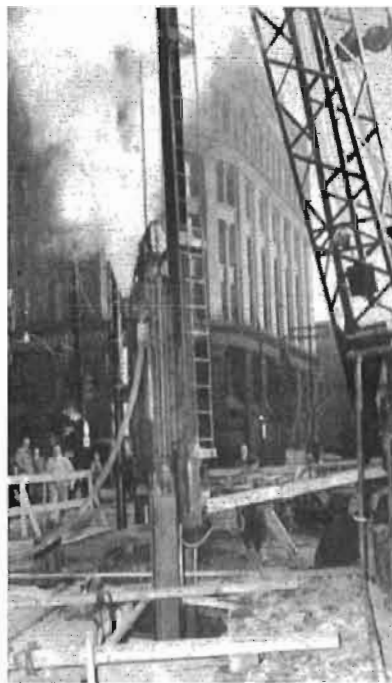
A pile driver in action on Front Street looking east, in the early stages of the work.
