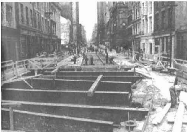
This photo illustrates the "cover" part of "cut and cover". It is taken on Yonge Street, looking north to Wellington, and shows the steel deck beams in place in the foreground, with timbering and laying of temporary street car tracks in the background.
