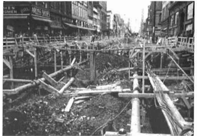
This view, looking north on Yonge Street from Albert Street, was taken on November 7, 1949. The numerous underground pipes and conduits are plainly visible.
