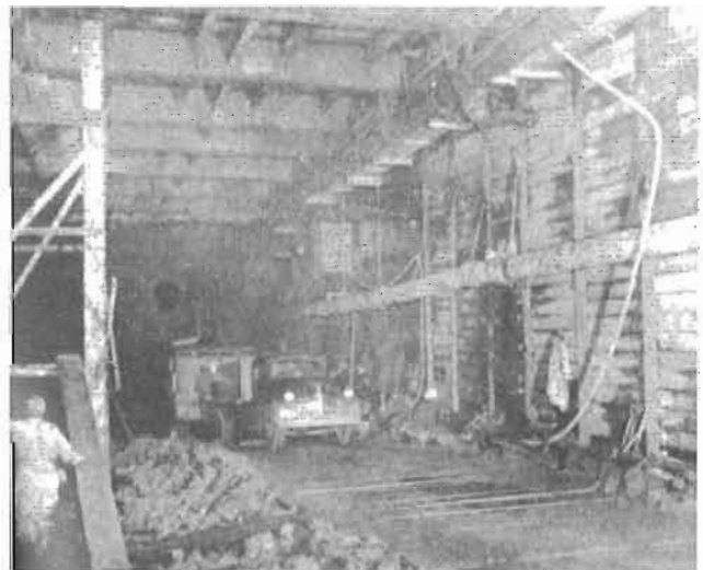
Excavation proceeded under the "cover". This photo shows the "intermediate lift excavation" in the area near Yonge and Queen. Heavy trucks are hauling earth up ramps to exits on side streets.
