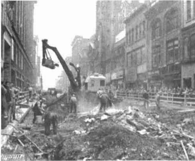
Excavation on Yonge Street, looking north from Queen. In the foreground air hammers are breaking up the soil.
