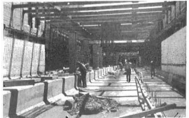
ABOVE: Concrete work progressing steadily in the area of Wellesley Station. Note the steel reinforcing bars ready to be placed in the concrete.
