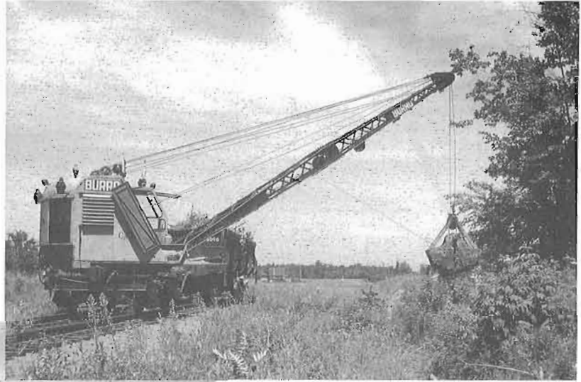
RIGHT AND BELOW: The first track into the museum site was built from the Candiac spur by the CPR. These two views were taken on June 28, 1962 and show the start of the work. In the background is the museum building under construction.
