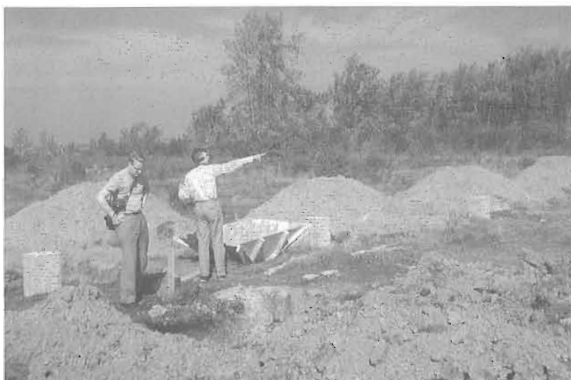
Paul McGee and Steve Cheasley looking over the site of the future museum on October 9, 1961. The contractor is already at work on the footings for the first building.
