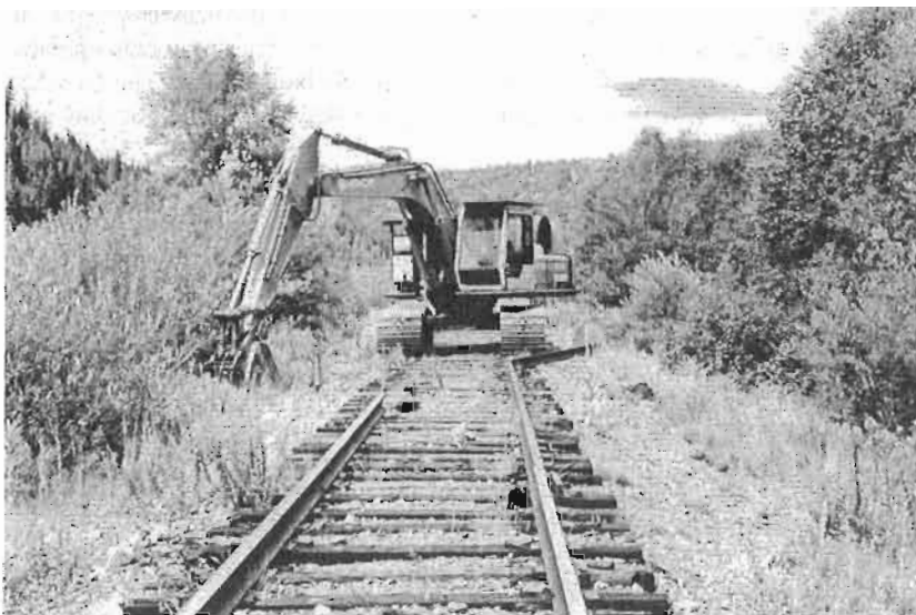
Excavator with magnet attached picking up rails from track and placing them to the sides of the right-of-way. Rails in foreground have had all their fastenings removed and are free standing.
