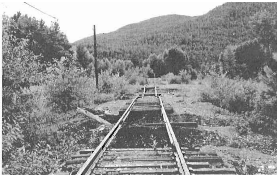
In mid 1991 almost all the track was in stable condition after passage of the last train two years before. This flood damage was an exception and was located between Coalmont [Mile 82] and Tulameen [Mile 86].
