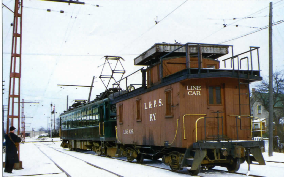
An overhead line problem on December 30, 1956 caused regular passenger service south of St. Thomas to be suspended for several hours. Car 10 and the line car were dispatched to fix the problem. After the problem was fixed, the repair train was caught departing St. Thomas near the Wabash RR station for the return trip to London. On this day there were only 7 weeks of passenger service remaining.
