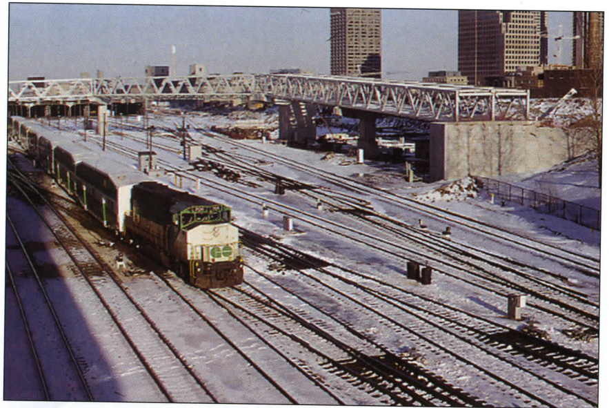
A westbound GO Transit commuter train eases out of Toronto Union Station on a wintry March 21, 1989. The structure under construction above the tracks is the pedestrian walkway connecting Union Station with the SkyDome, which opened in June 1989. CRHA Archives, Fond Bury No. CDN(m)3-123.
