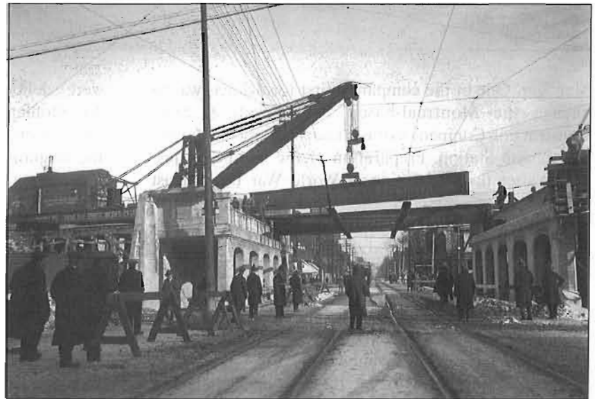
Construction on the viaduct began in the east near Logan Avenue and extended west towards Union Station. There appear to be more officials than workers in this 1926 view showing the Queen Street subway under construction. City of Toronto Archives, Series 372, Sub-Series 79, Item 160
