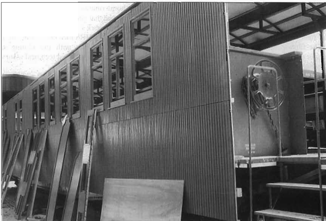
One of the two open cars belonging to Kamloops Heritage Railway being fitted with panels to convert it into an 1880s coach, the conversion being made only on its north side. View taken at KHR private yard in Kamloops, BC, at end of May 2007. All photos by the author.
