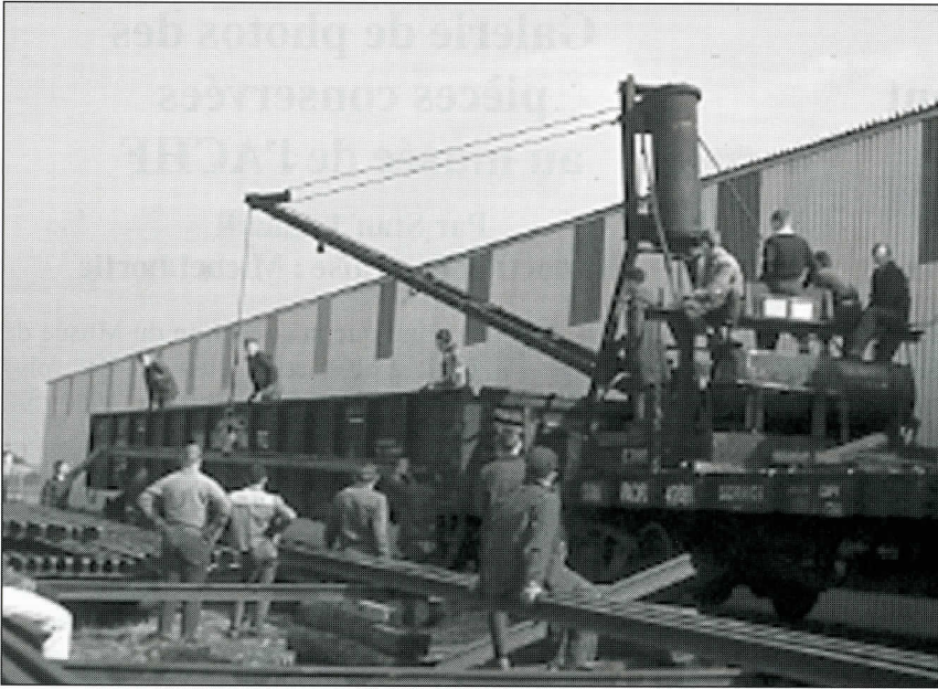
It is easy to remember the ‘mechanical assists’ that arrived on site in those early years, first was the air compressor and pneumatic spike driver; then the number 9 switcher. In 1964 the CPR donated an air hoist mounted on a flat car, this was a invaluable in handling rails and other heavy items to this day. CRHA Archives, Fond Angus # 5122.
