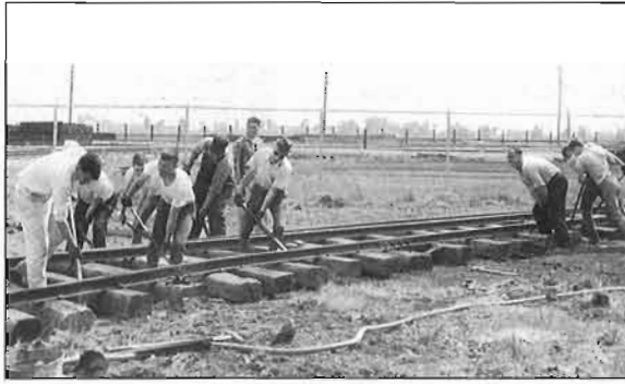
'Heave Ho' as volunteers align track leading into Building One. From left to right are Fred Angus, Dennis Peters, James Sandilands, Ron Bryant, C. Stephen Cheasley and Omer Lavallee at right. CRHA Archives.
